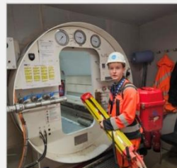
Marcelina Klimek Entering the pressure chamber for surveying a tunnel in an urban railway project that is constructed under compressed air at 2300mb - a strange feeling every day.
